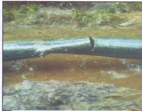
Affected section of facility
